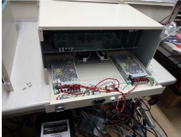
Figure 9: Pulling out the power supply board
