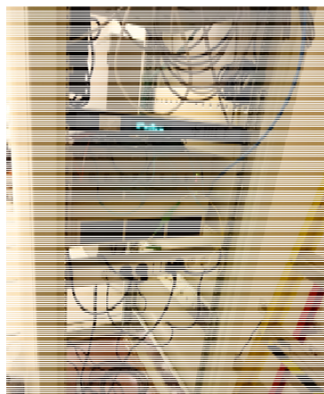
Figure 1 OFL MUX installed onto the in the correlator room at the AOS.
