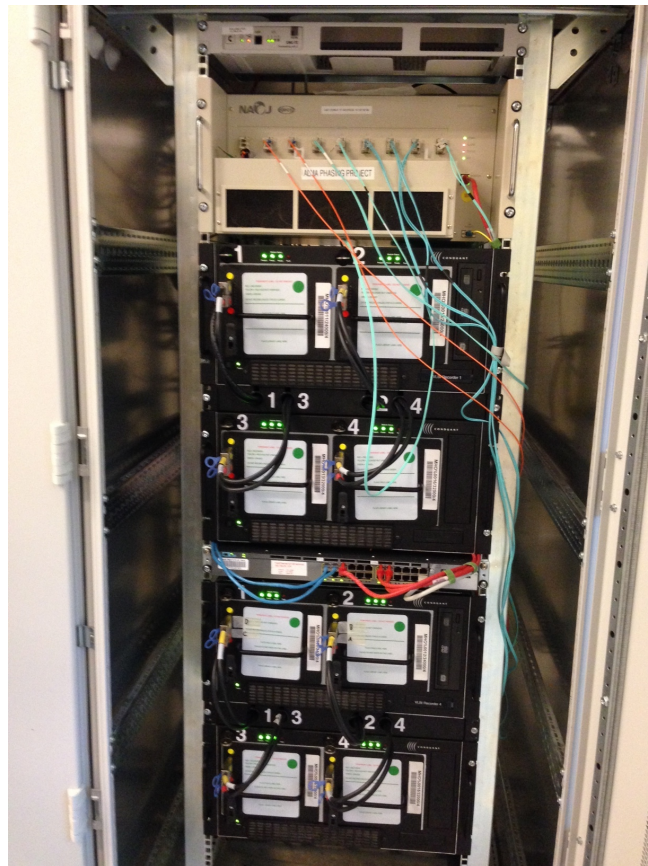
Figure 3.1: Recorders 1 and 4 installed in the designated OSF computer room rack. The OFLS demux unit is at the top. Between the recorders is the network switch which connects the recorders to the AOS net and also provides a private network between the recorders.
