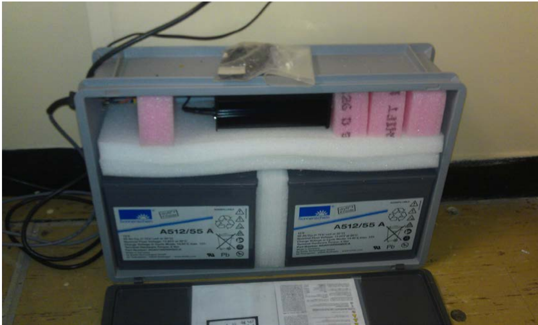
Figure 3-9: Photo of H-Maser UPS battery assembly
