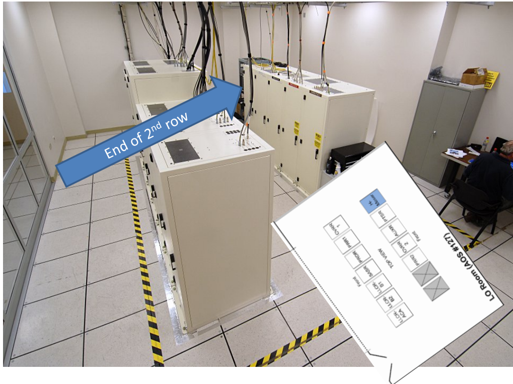
Figure 3-2: Photo of CLOA Racks with intended position of H-Maser indicated, as well as the location of the unused rack slots
