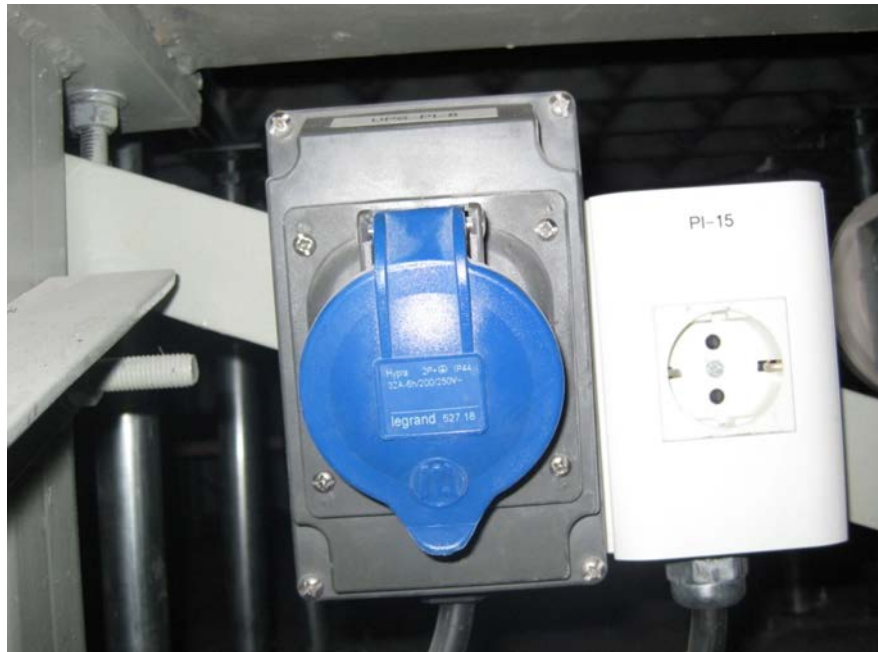
Figure 3-5: Receptacles provided for the H-maser
