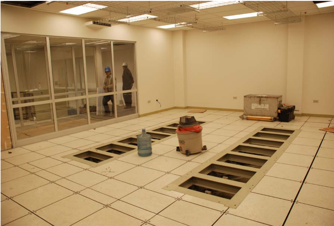
Figure 3-3: LO room floor before racks installation showing: outline of isolated pad, seismic support structure, bolt patten, and AC power receptacles
