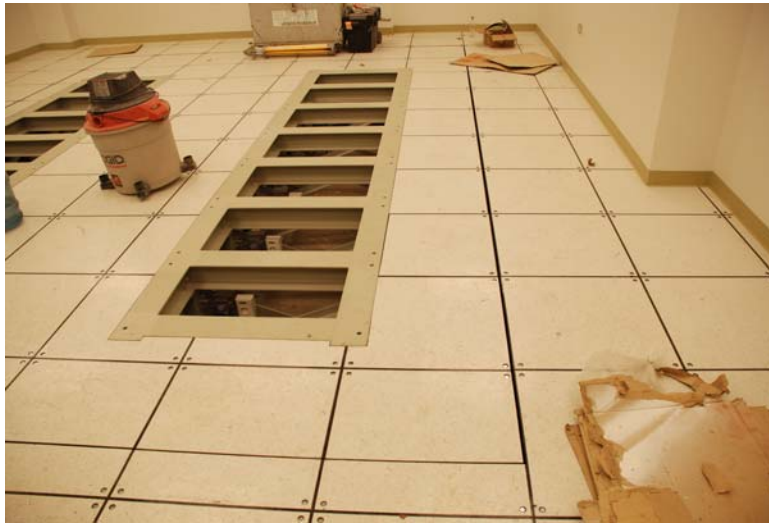
Figure 4 - Photo of the installed seismic support with the computer floor installed flush with the top surface
