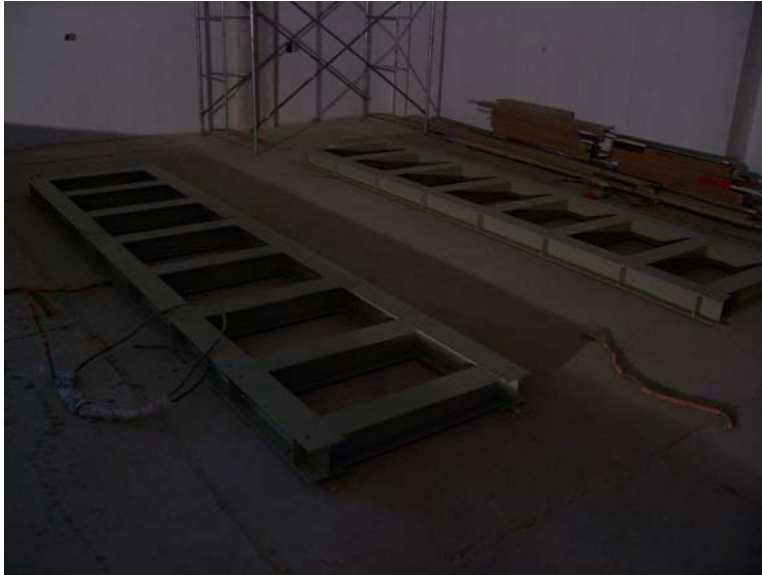
Figure 2 - Frame of Seismic support structure shown laid out on top of the isolated slab prior to installation
