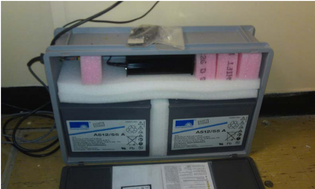
Figure 8 - Photo of H-Maser UPS battery assembly
