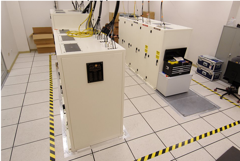
Figure 5 - Final installation of Central LO racks
